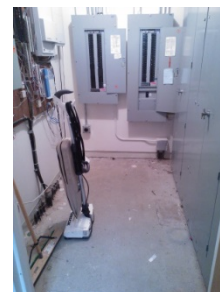
Electrical closet cleared of all items bringing our building within fire code standards.
